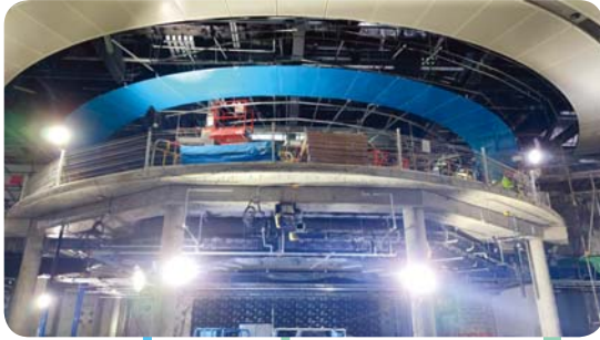
Three Runway System Project - New Integrated Airport Centres - Building and Civil Works
