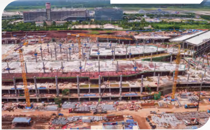
The concrete structure of the Terminal 2 was capped. T2航站楼混凝土結構封頂。
