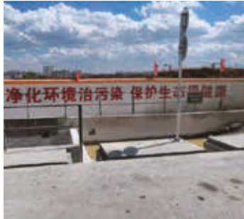
Tertiary sedimentation tanks for waste slurry and wastewater 廢漿水三級沉澱池
