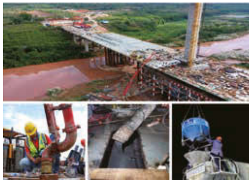
The first enterprise in Yunnan Province to achieve local industrialisation application of ultra-high performance concrete 雲南省首家實現超高性能混凝土本土產業化應用的企業
