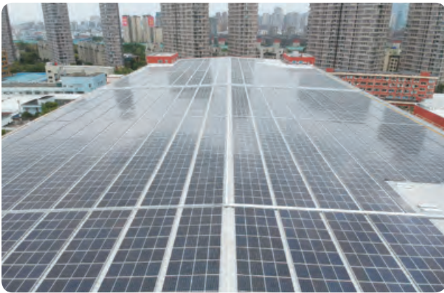
寧波廠區的太陽能發電板 PV panels in the Ningbo factory area
