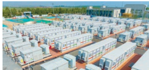
Haiyang Energy Storage Power Station
