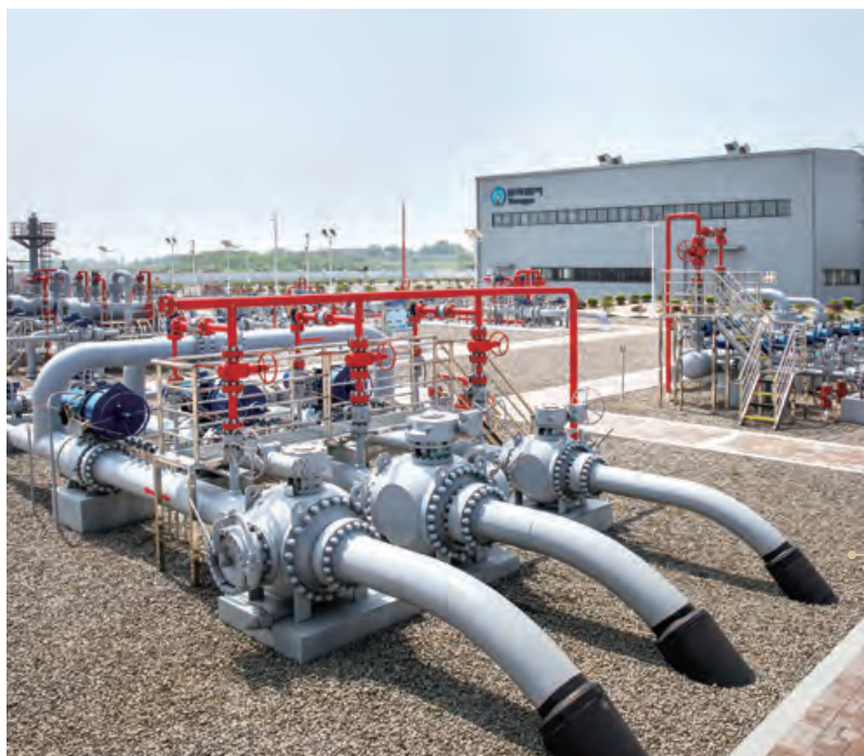
In Jintan, Changzhou, Jiangsu province, we operate an underground gas storage facility with increasing peak-shaving capability.
