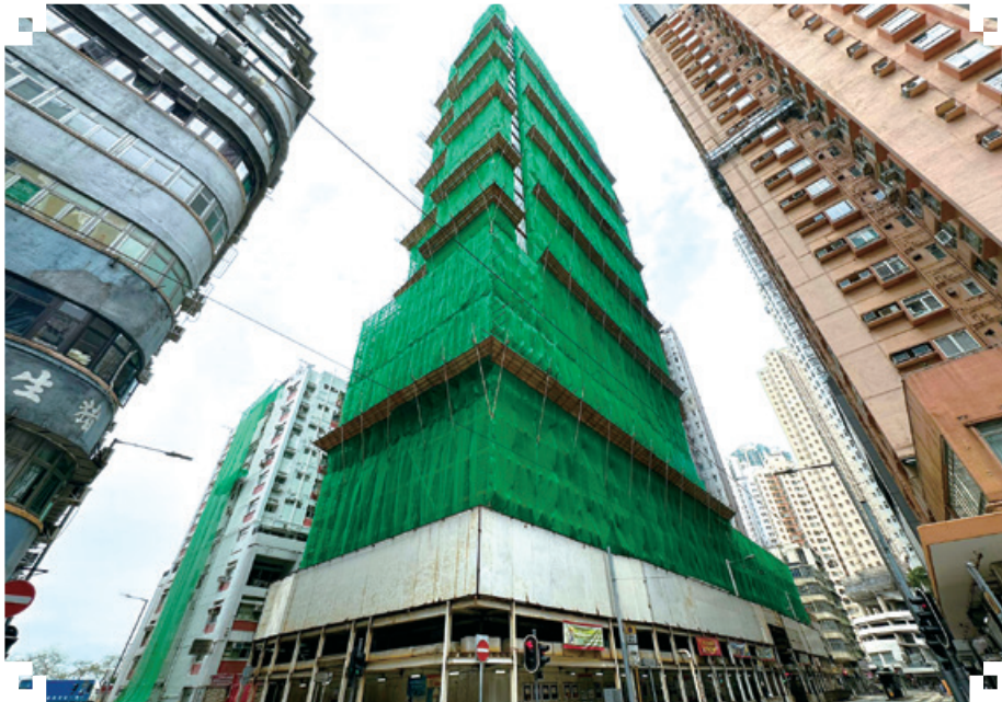
Proposed residential and commercial development at Nos. 33-47 Catchick Street, Kennedy Town 堅尼地城吉席街33號至47號之建議住宅及商業發展項目
