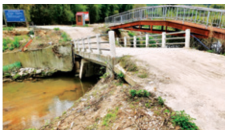
A dangerous bridge damaged by flood
