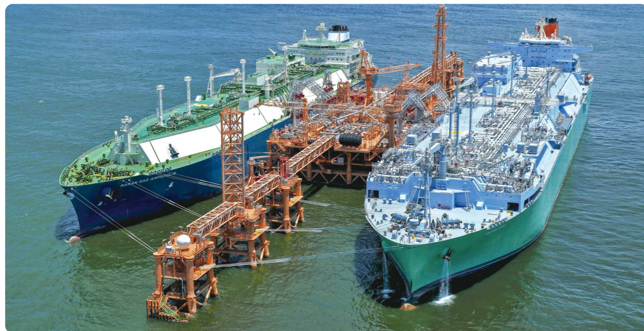
HK Electric, in partnership with the other power company in Hong Kong, commissioned Hong Kong’s first Offshore LNG Terminal in July 2023.
