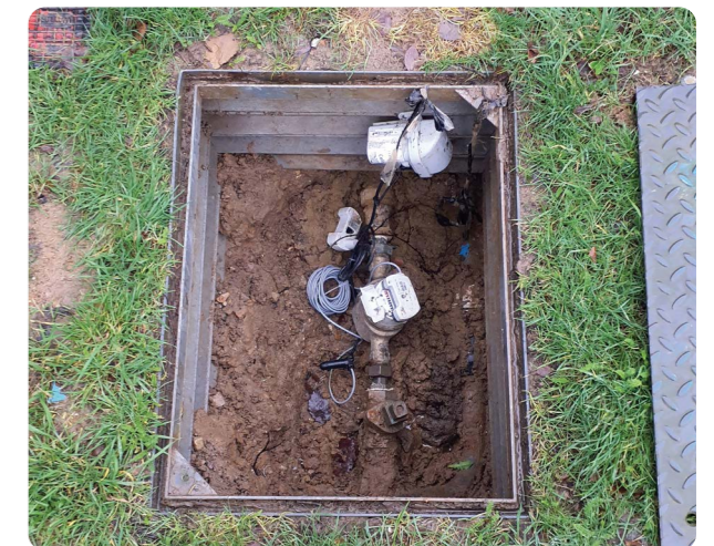
UKPN installs new Automatic Meter Readers to monitor water consumption.
