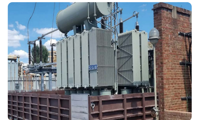
Permanent flood barriers protect the site against the prospect of a 1-in-1,000 year flood of the River Wandle.
