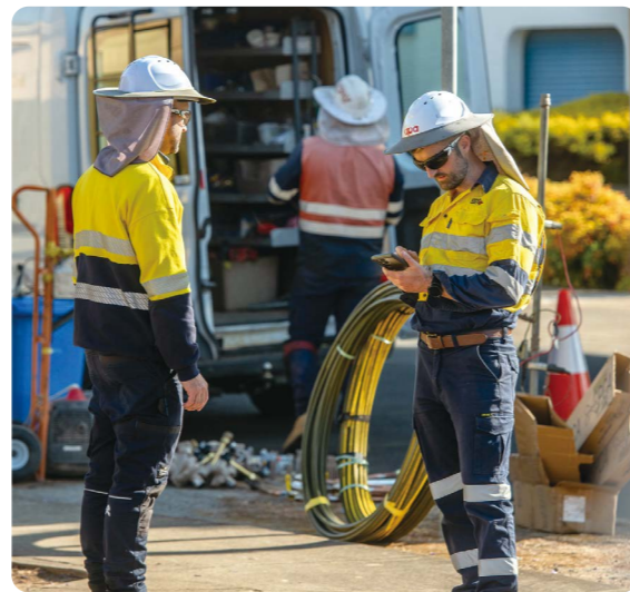
AGN’s Mains Replacement Programme has the added benefit of achieving emissions reductions in the near term and ensures our network is ready for hydrogen in the future.
