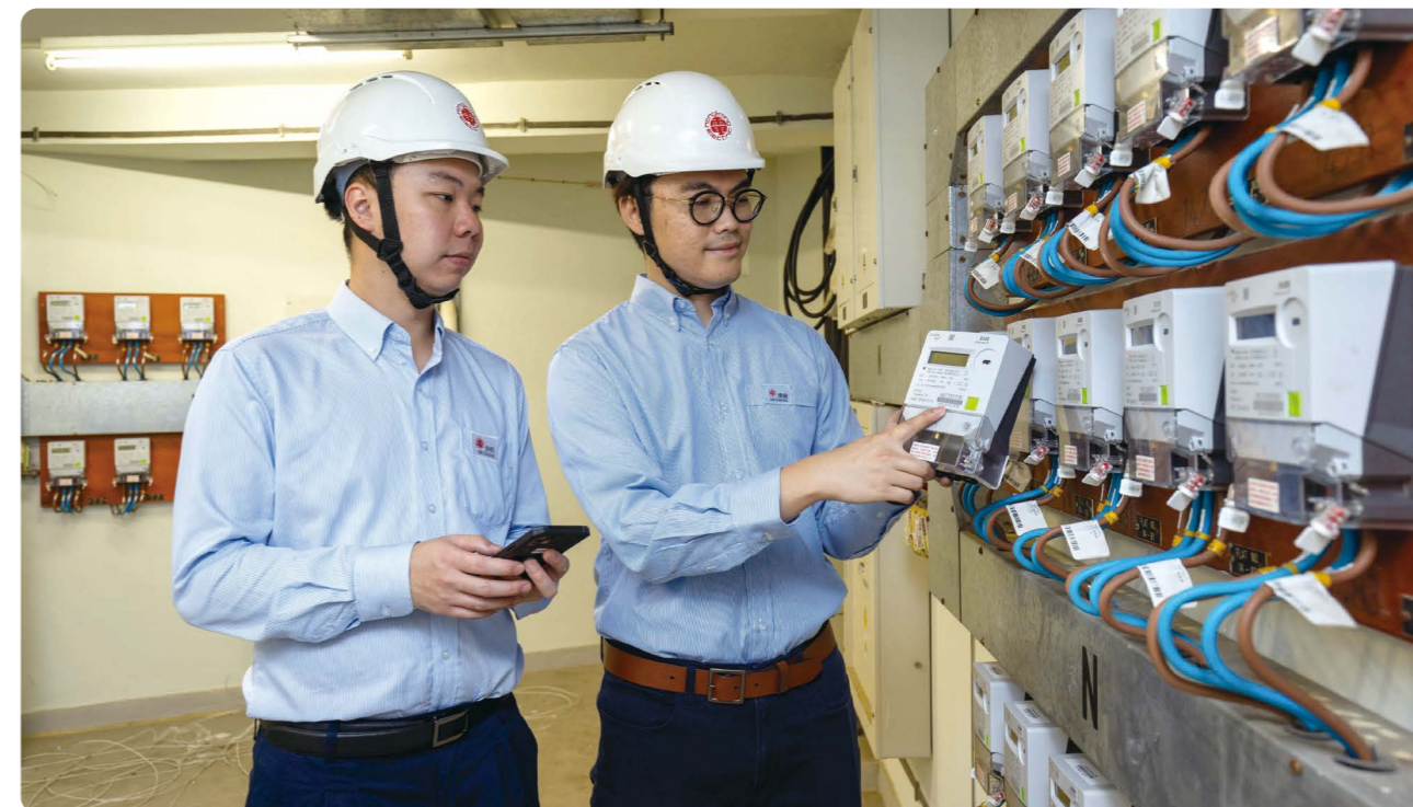
Over 580,000 customers will be involved in the deployment of Smart Meters, allowing them to further optimise their energy use more effectively.
