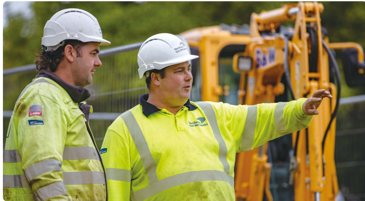
NGN helps biomethane producers get their gas into our grid, through a comprehensive support service.
