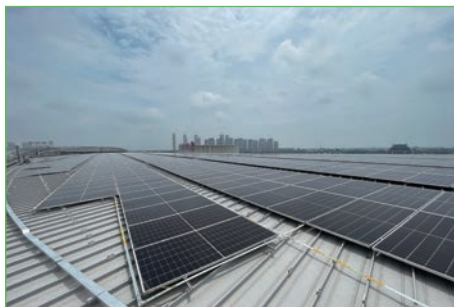
Wuxi Bonski Rooftop Photovoltaic – Completed
