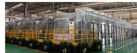
低溫乾化系統 Low Temperature Drying System
