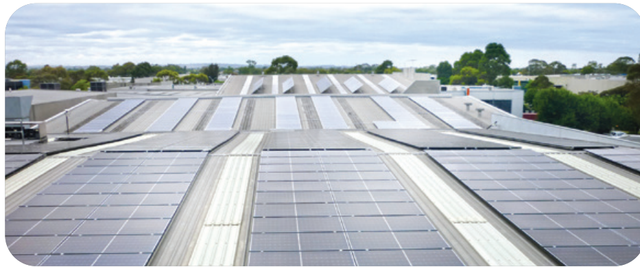
Solar panels implemented in Keysborough Site
