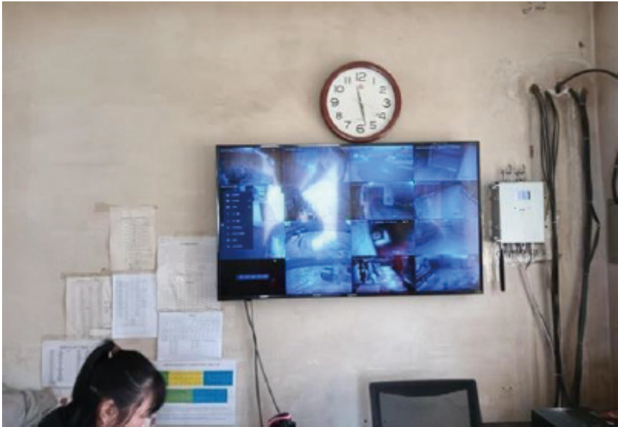
Figure 15-4 Control room monitoring the underground workings and access gates
