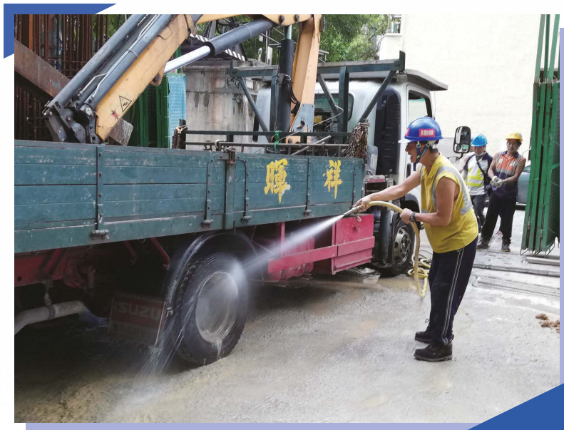
Designated wheel washing area at site 於地盤設立指定輪胎清洗區
