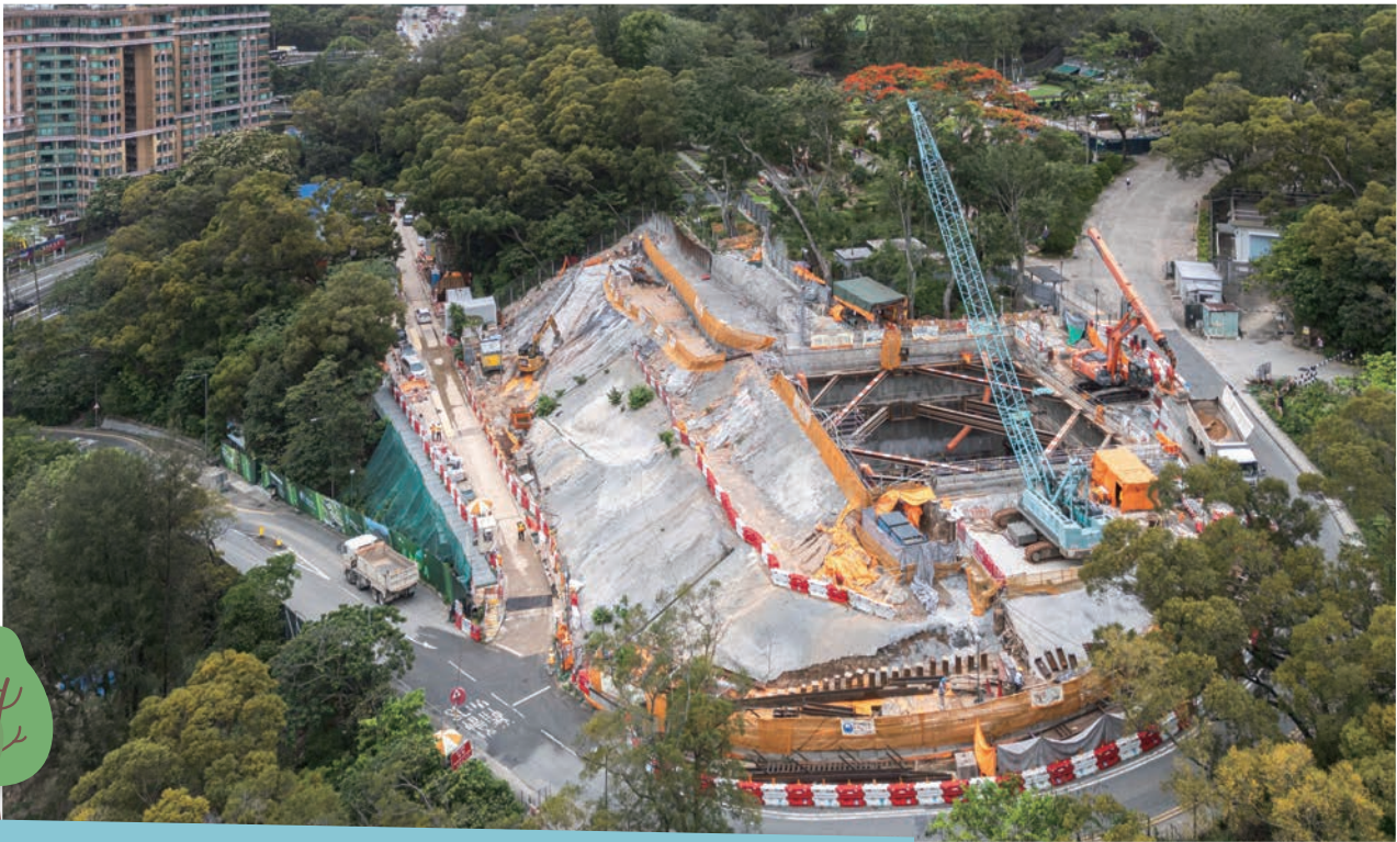
Relocation of Diamond Hill Fresh Water and Salt Water Service Reservoirs to Caverns 搬遷鑽石山食水及海水配水庫往岩洞
