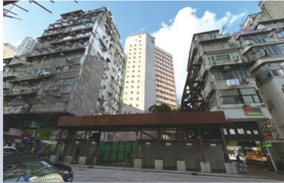
Castle Peak Road re-development project site at Sham Shui Po 深水埗青山道重建項目地盤
