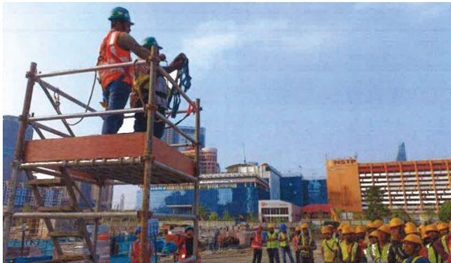
The Grand ToolBox awareness on “Safety Harness and Working at Height” at project site on 23 February 2024.
